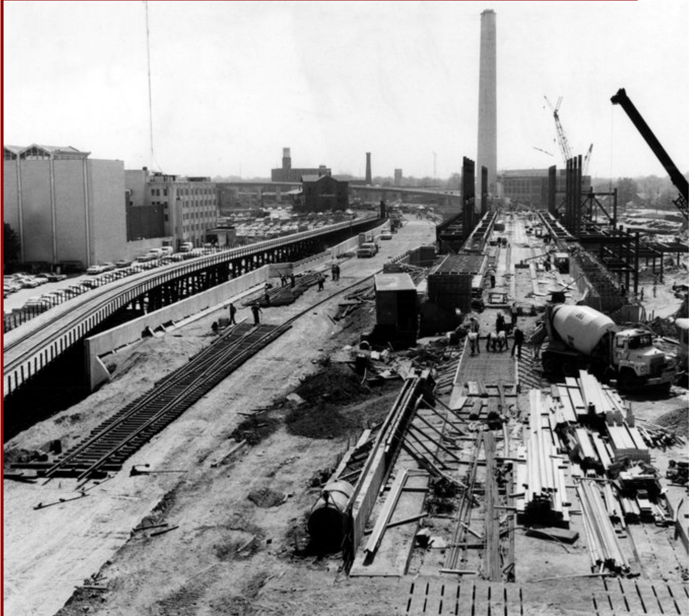
A MARTA station under construction on the edge of downtown Atlanta, 1978. Charles Pugh/Atlanta Journal Constitution, via Associated Press
